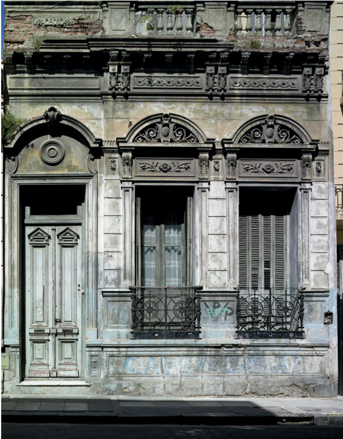
Classical Revival facade, San Telmo neighborhood; Buenos Aires, Argentina; 2006; photograph © Richard Sexton
